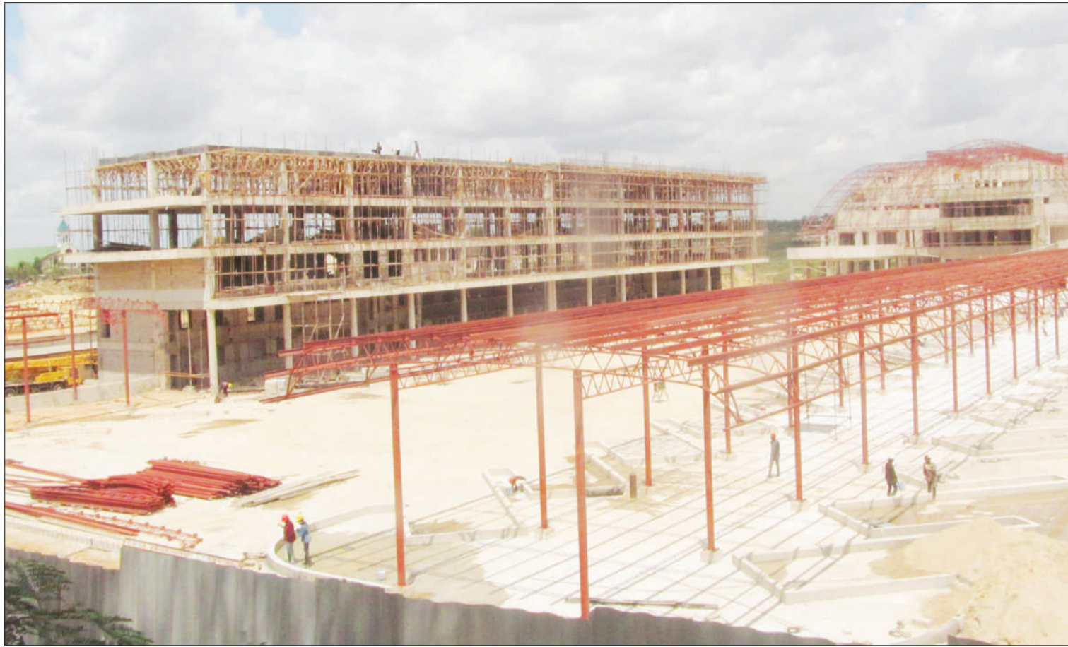
This is how the modern long-distance commuter bus terminal under construction at Mbezi Mwisho in Dar es Salaam now looks, as captured by correspondent Sabato Kasika yesterday. It has been reliably learnt that it is expected to become operational later this year, taking over from the one at Ubungu.
