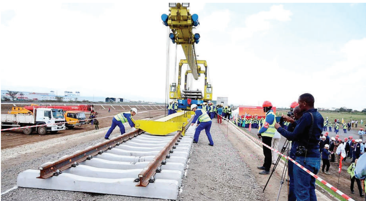
Workers lay tracks for the standard gauge railway phase 2A at Suswa section in Narok, Kenya
