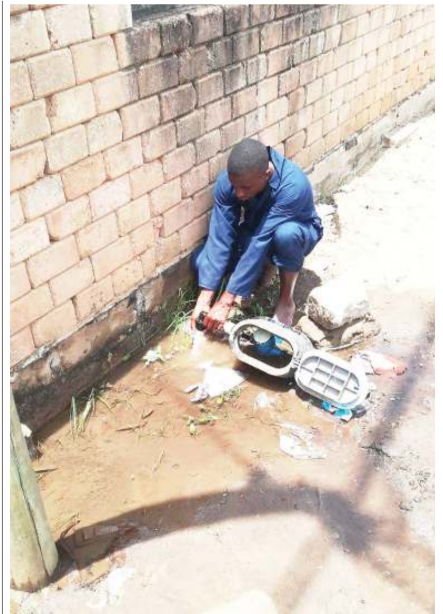
Dar es Salaam Water and Sewage Authority employee repairs a leaking pipe leading to a customer's residence in Dar es Salaam's Boko suburb yesterday. Photo: Guardian Correspondent
