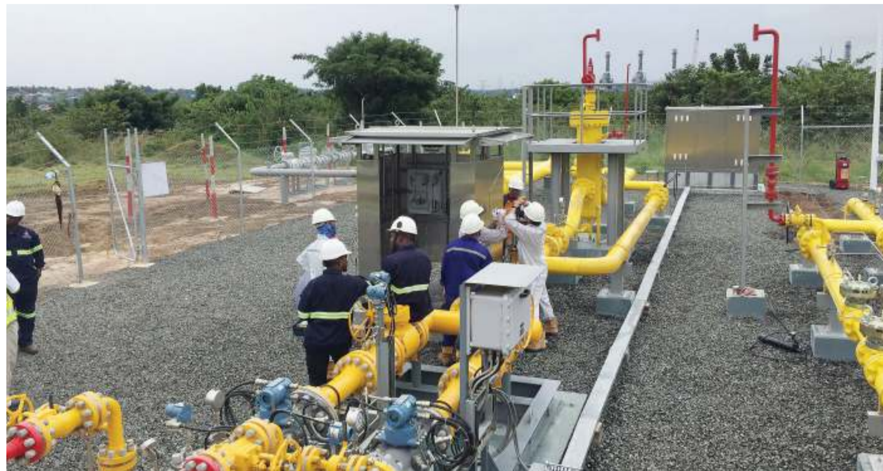
CPP and Tanesco engineers install pressure reducing station at Kinyerezi I gas power supply plant in Dar es Salaam earlier this week. Photo: Correspondent Prosper Makene.
