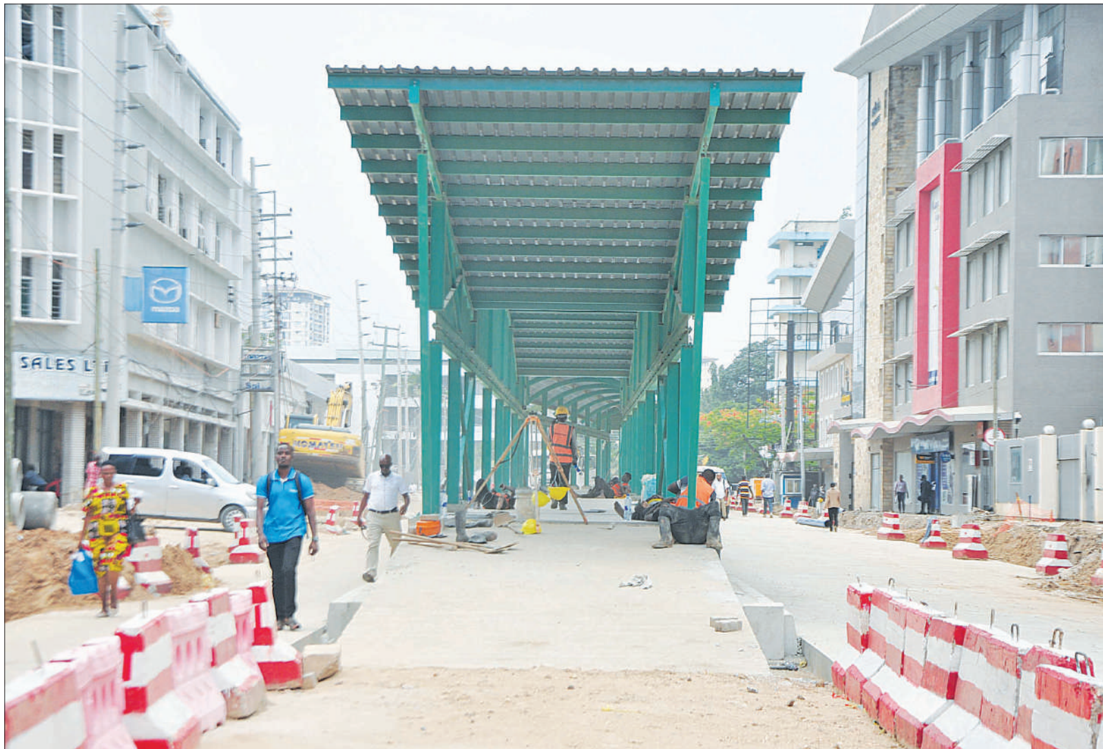
A view captured yesterday of the Bus Rapid Transit (BRT) station at the Old Post Office section of Sokoine Road in downtown Dar es Salaam city, with implementation of the ambitious project ongoing. Photo: Correspondent Imani Nathaniel
