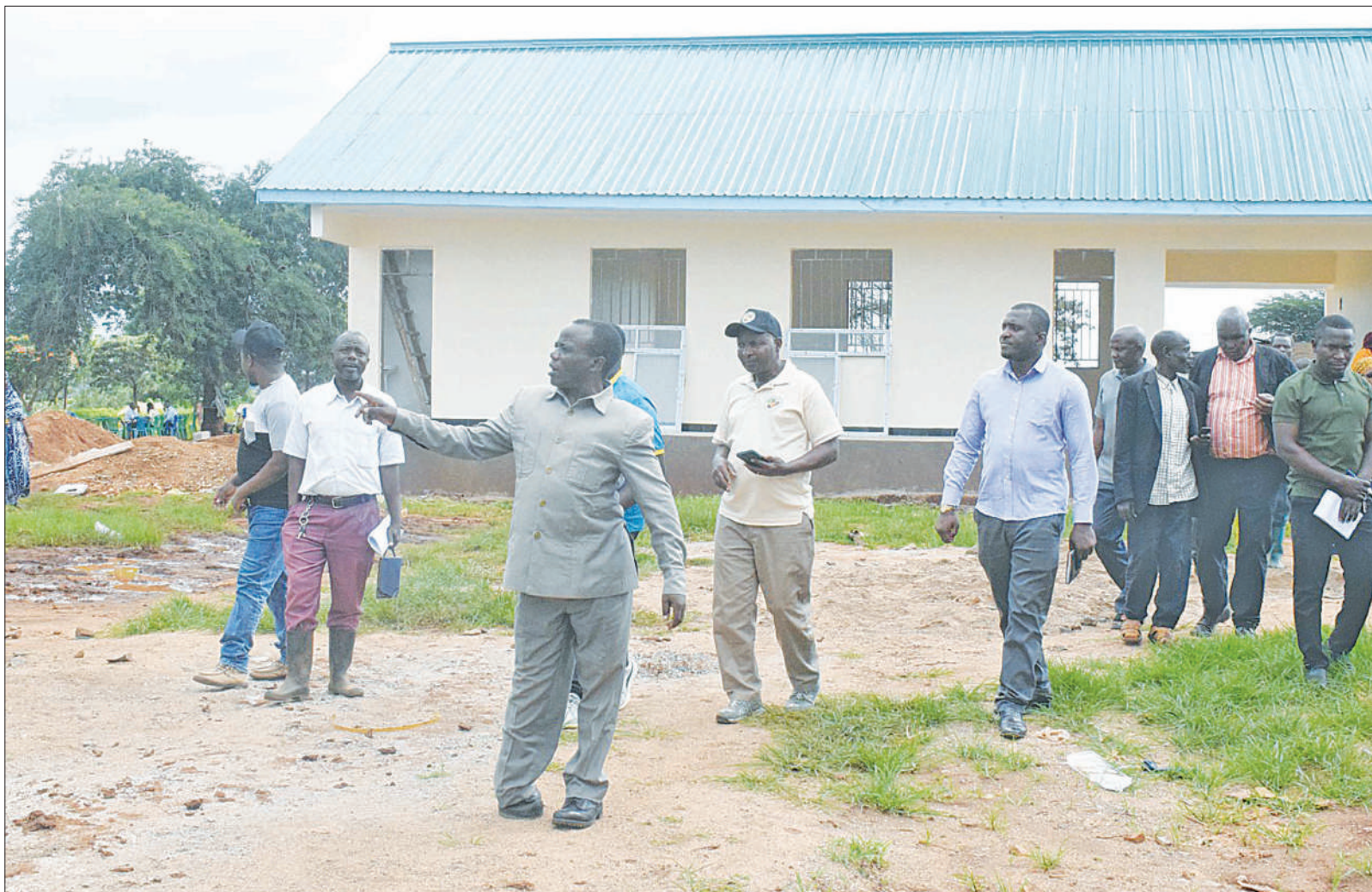
James Mkwega (foreground, gesturing), Chairman of the Mkalama District Council in Singida Region, pictured earlier this week leading members of the council's Planning, Finance and Administration Committee on an inspection tour of progress in the construction of Kidarafa Secondary School in Mwangi ward. Photo: Correspondent Tobias Mwanakatwe
