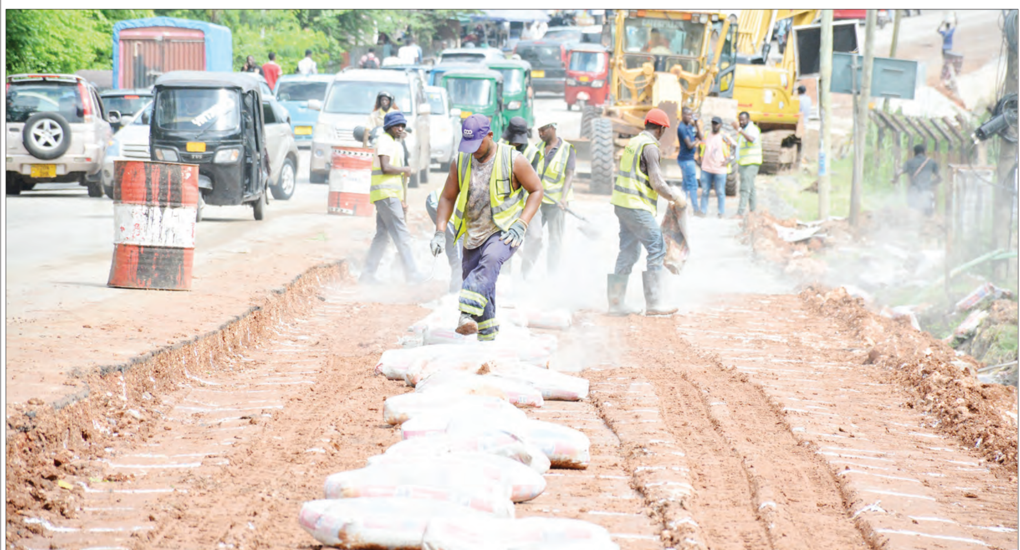
Expansion work on the road stretch from Mlimani City shopping complex to the University of Dar es Salaam, up to the Sam Nujoma Road junction close to the Water Resources Institute being carried out yesterday. It is meant to reduce congestion of vehicles and prevent accidents. Photo: Correspondent Miraji Msala
