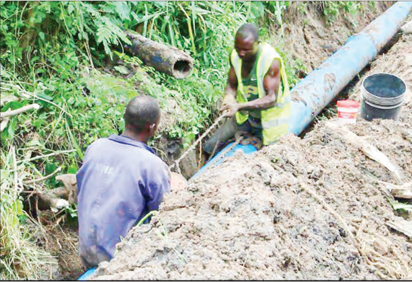
Dar es Salaam Water and Sanitation technicians laying water pipes at Golani, Kimara ward in Ubungo being part of the implementation in accessing domestic water supply. Photo: Guardian Correspondent
