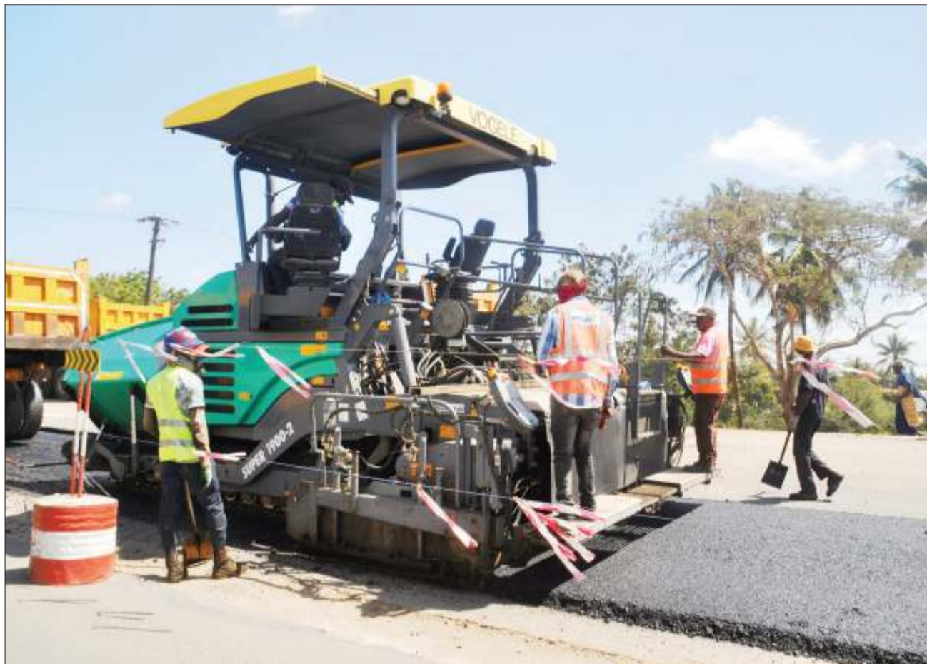
Estim construction workers at work along Morogoro Road section of Kimara - Kibaha of a dual carriageway phase one including the construction of Kibamba, Kiluvya and Mpji bridges as captured by our photographer at Kimara Temboni in the outskirts of Dar es Salaam yesterday. Photo: John Badi
