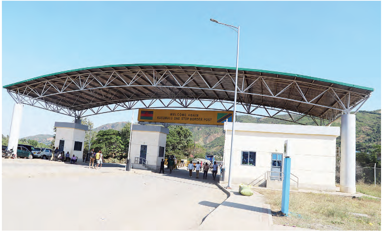
This is a scene from the Kasumulu One-Stop Border Post offices still undergoing construction at the Tanzania-Malawi border in Kyela District, Mbeya Region, as captured yesterday. Photo: Correspondent Shukuru Senkondo
