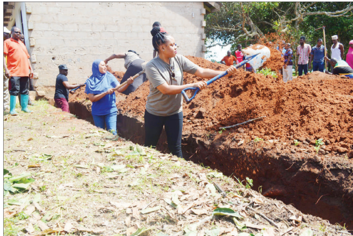
Kisarawe district commissioner Jokate Mwegelo (R) takes part in the digging of a foundation pending the construction of classroom building at Jengu Secondary School yesterday. Photo: Guardian Correspondent
