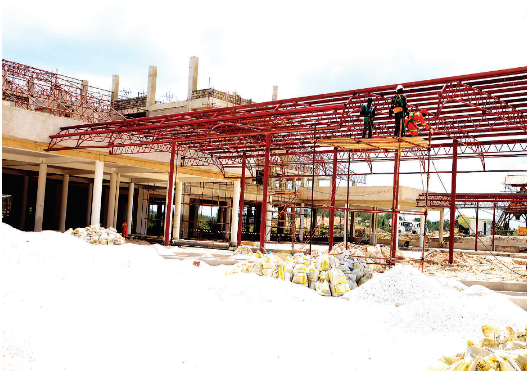
Work in progress at the site of what is meant to be a modern long-distance bus terminal - at Mbezi Luis in suburban Dar es Salaam - as found yesterday. Photo: Correspondent Jumanne Juma
