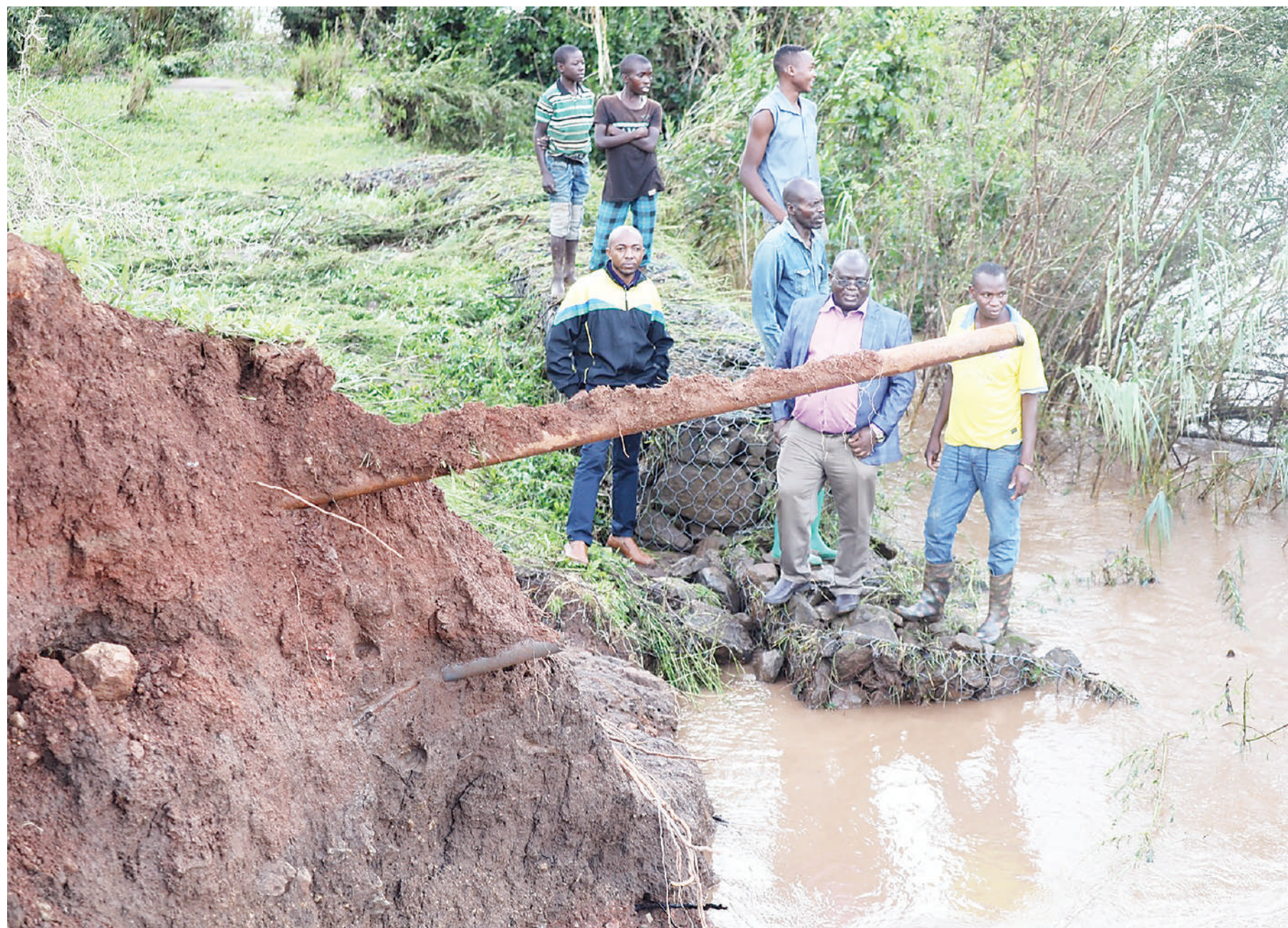
Works and Transport deputy minister Godfrey Kasekenya (2nd R) during a visit to inspect a bridge linking Ilulu and Chagu villages which had been swept away by flood waters in Ileje District, Songwe Region recently. Photo: Guardian Correspondent Siti Said
