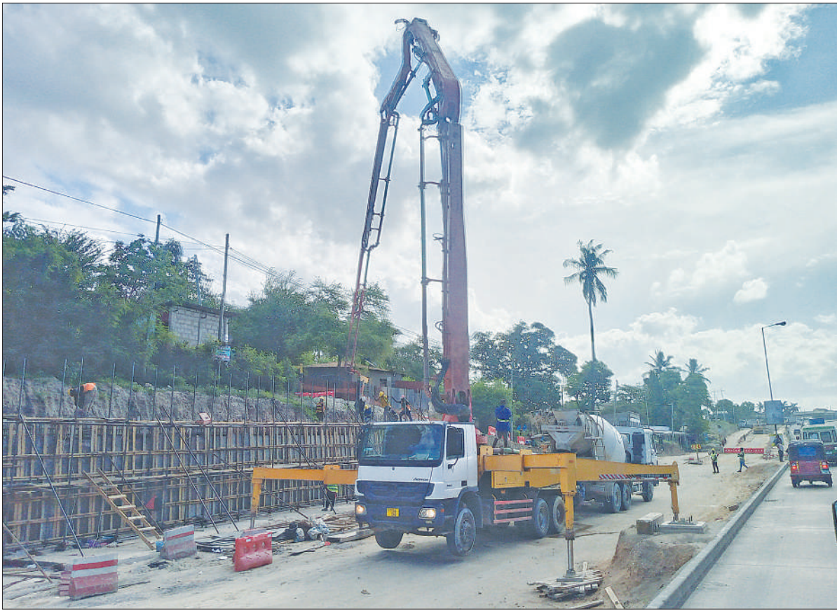
Morogoro Road expansion in the city of Dar es Salaam is making progress, as seen in the Kimara Corner section yesterday. The works are meant to ease traffic congestion and improve connectivity from the city centre to the suburbs. Photo: Correspondent Sabato Kasika
