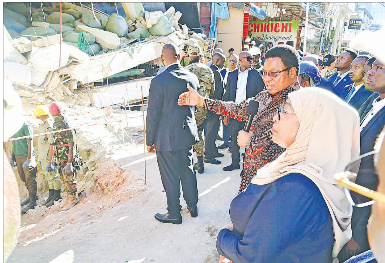
President Samia Suluhu Hassan receives listens to Prime Minister Kassim Majaliwa when visiting the site of the building collapse disaster at Kariakoo business zone in Ilala District, Dar es Salaam Region yesterday. Photo: State House
