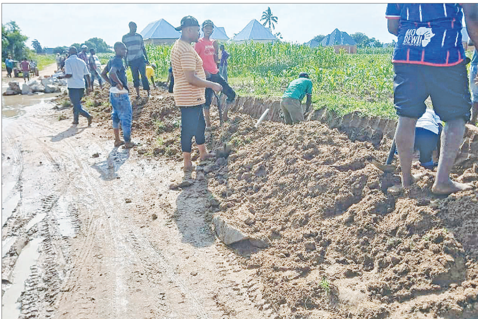
Residents of Mhongolo ward in Kahama municipality pictured yesterday digging a drainage canal, primarily in a bid to tame seasonal floodwaters. Photo: Correspondent Shaban Njia
