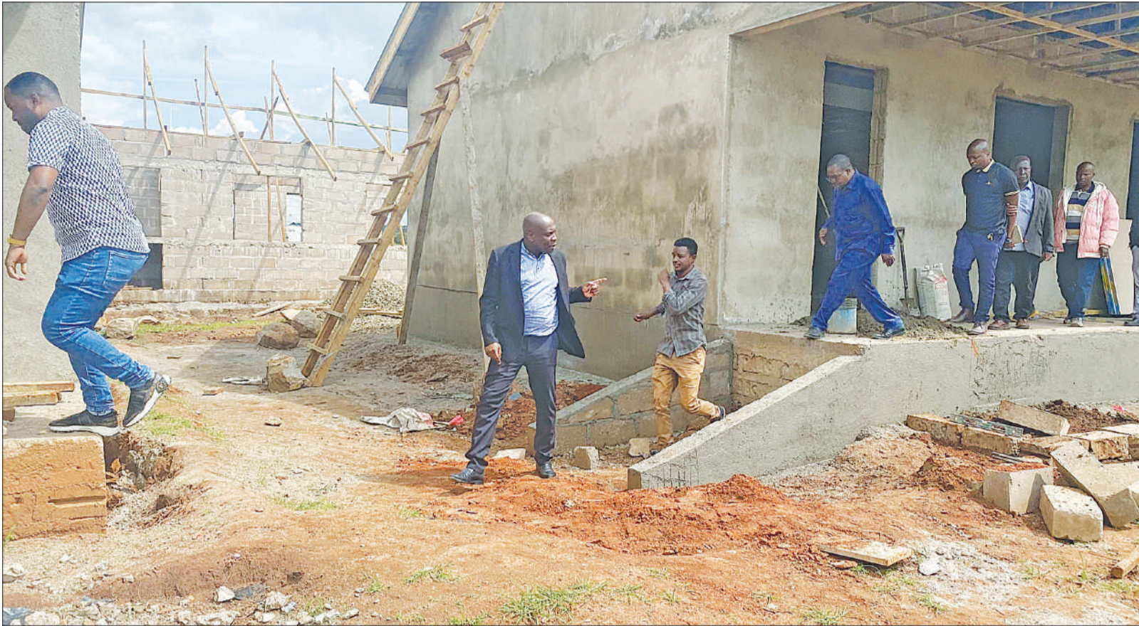
Mkalamla district commissioner Moses Machali (6th-R) leads the inspection of progress in the construction of buildings at Kidarafa Secondary School. The completion of the project will spare students in the area the need to travel a daily 14 kilometers from home to school and back to attend classes at the school nearest their residences. Photo: Correspondent Thobias Mwanakatwe
