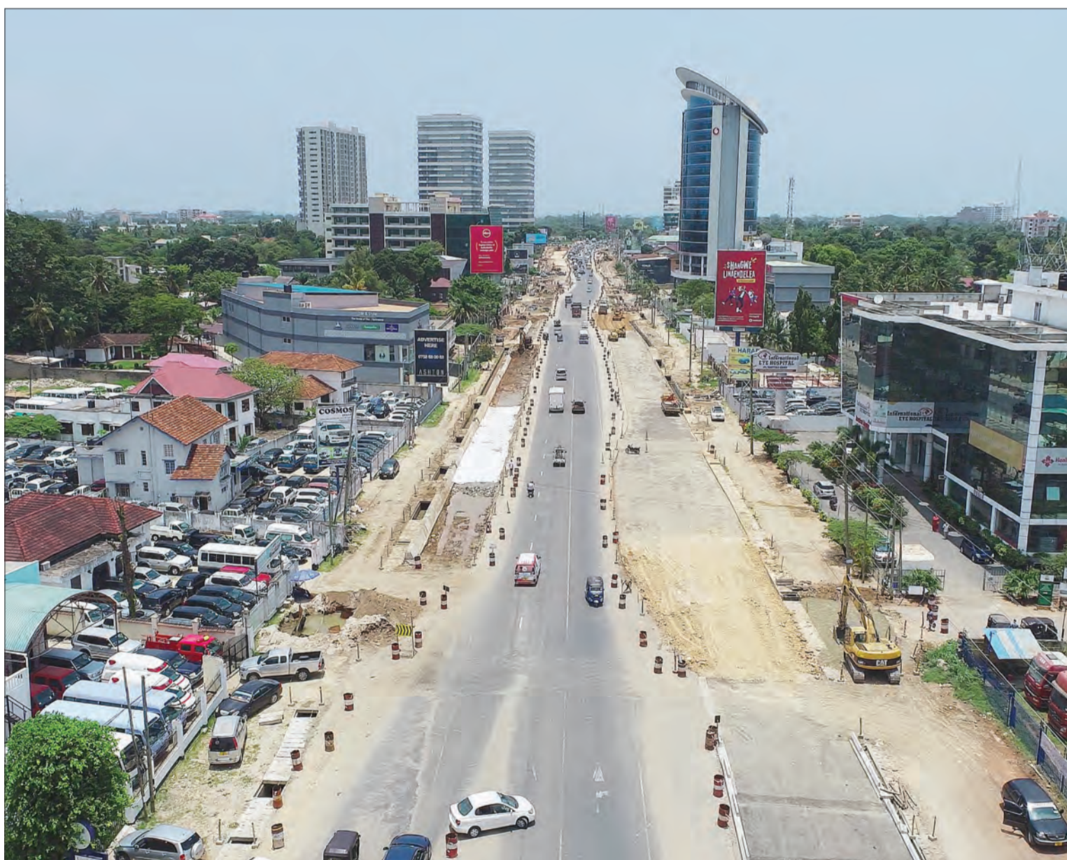
This is a scene from a section of the Morocco-Mwenge stretch of Dar es Salaam's Ali Hassan Mwinyi Road, whose expansion is reported to have reached 70.35 per cent. It was captured yesterday. Photo: State House
