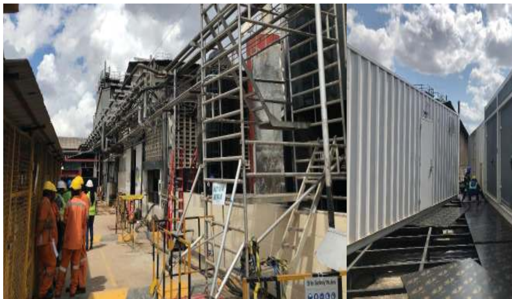
SBL's ongoing construction works for the expansion of Dar plant that started early this year. Photo: courtesy of SBL.
