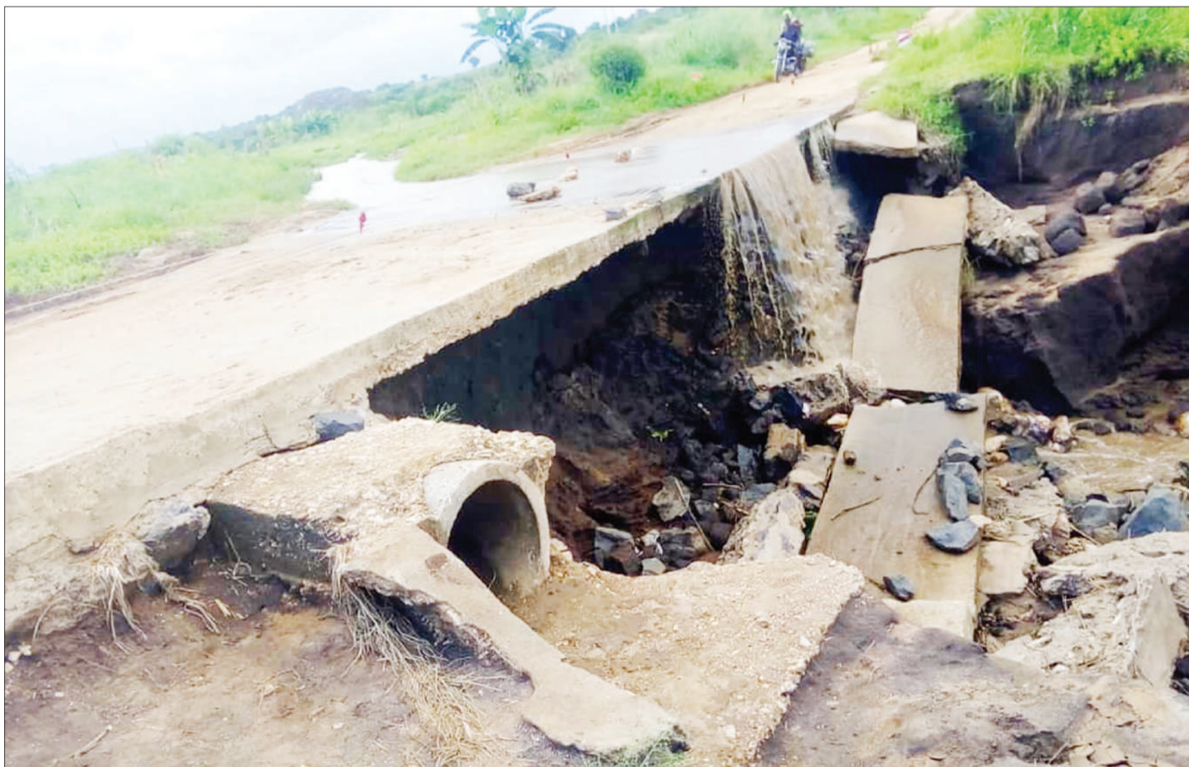
Kwamasimba bridge, which lies in Kilindi District's Kiburashi ward, in grave danger of collapse in the wake of weeks of relentless pounding rains. Photo: Correspondent Boniface Gideon
