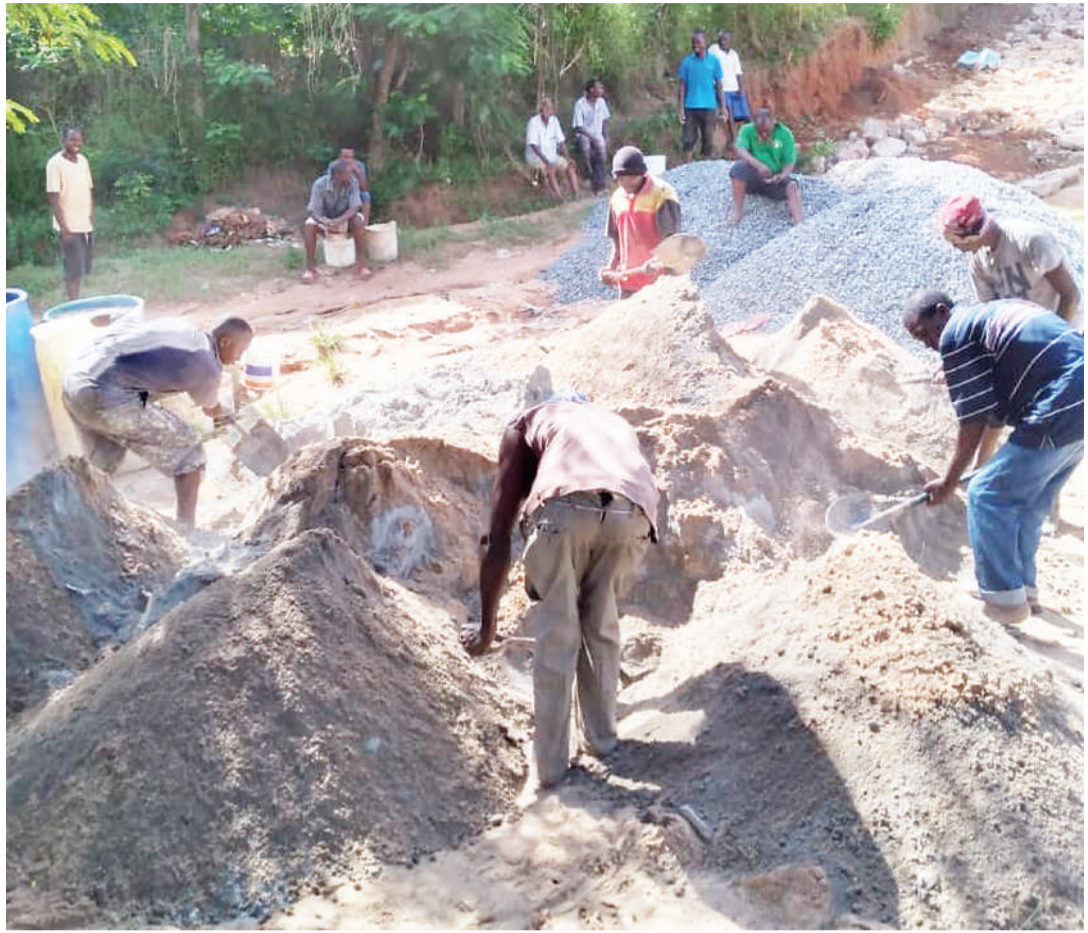
Residents of Tabata Kisukuru in Ilala District, Dar es Salaam, participate in the rehabilitation of a feeder road on self-help basis - as found at the weekend. Photo: Correspondent Joseph Mwendapole
