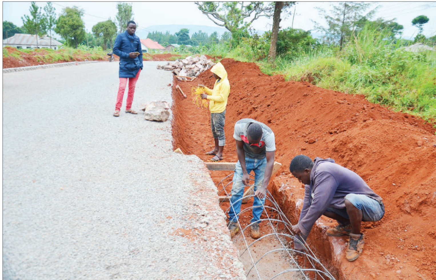
Work in progress on drainage system along a newly rehabilitated trunk road in Muleba District, Kagera Region, as found yesterday. Photo: Correspondent Jumanne Juma
