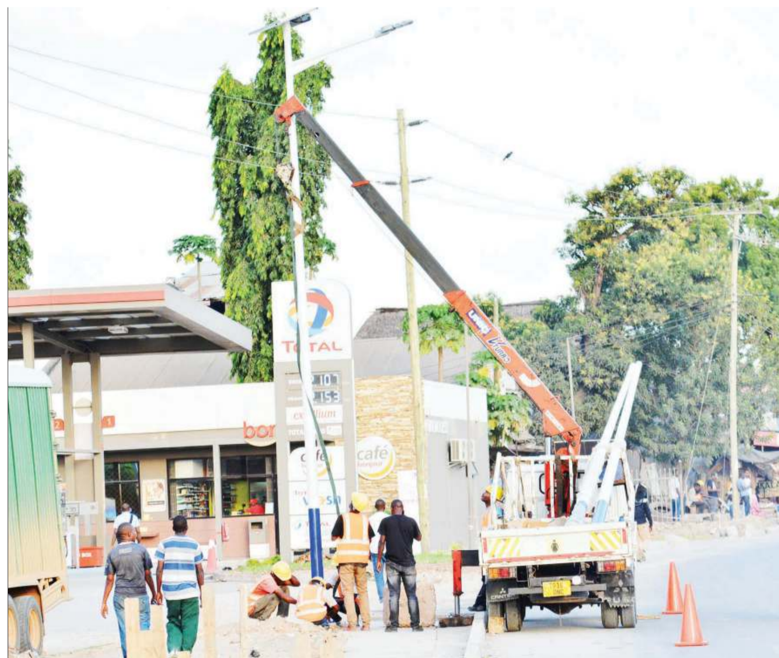
Technicians install a solar power pole at Temeke kwa Sokota in Dar es Salaam at the weekend. Photo: Correspondent Miraji Msala
