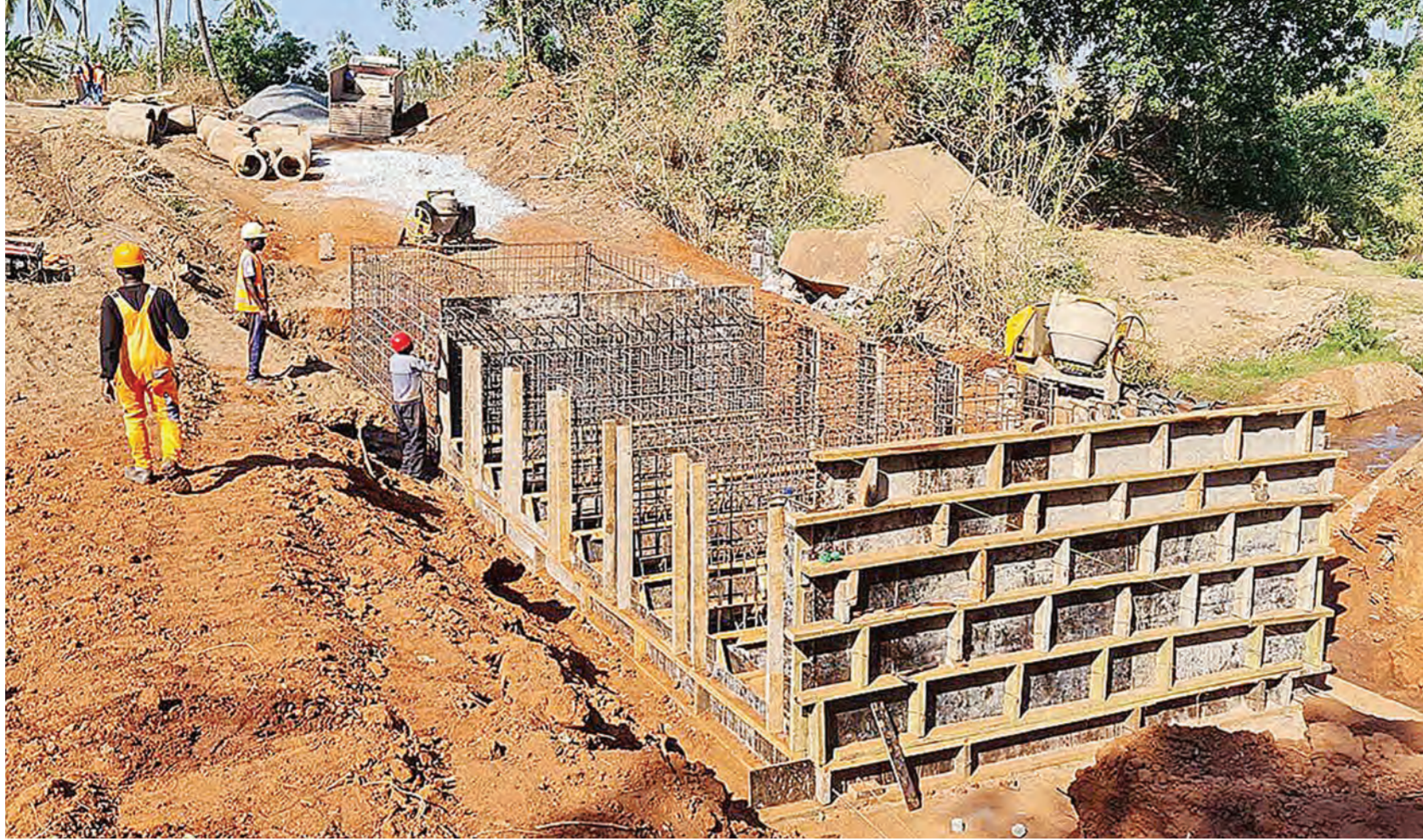
TNR Engineering kicked off work for the Lindi Jumbo graphite project in late August last year beginning with a bridge required for crossing a river crossing to the site. The work was undertaken under the supervision of the Tanzania National Roads Agency (TANROADS)
