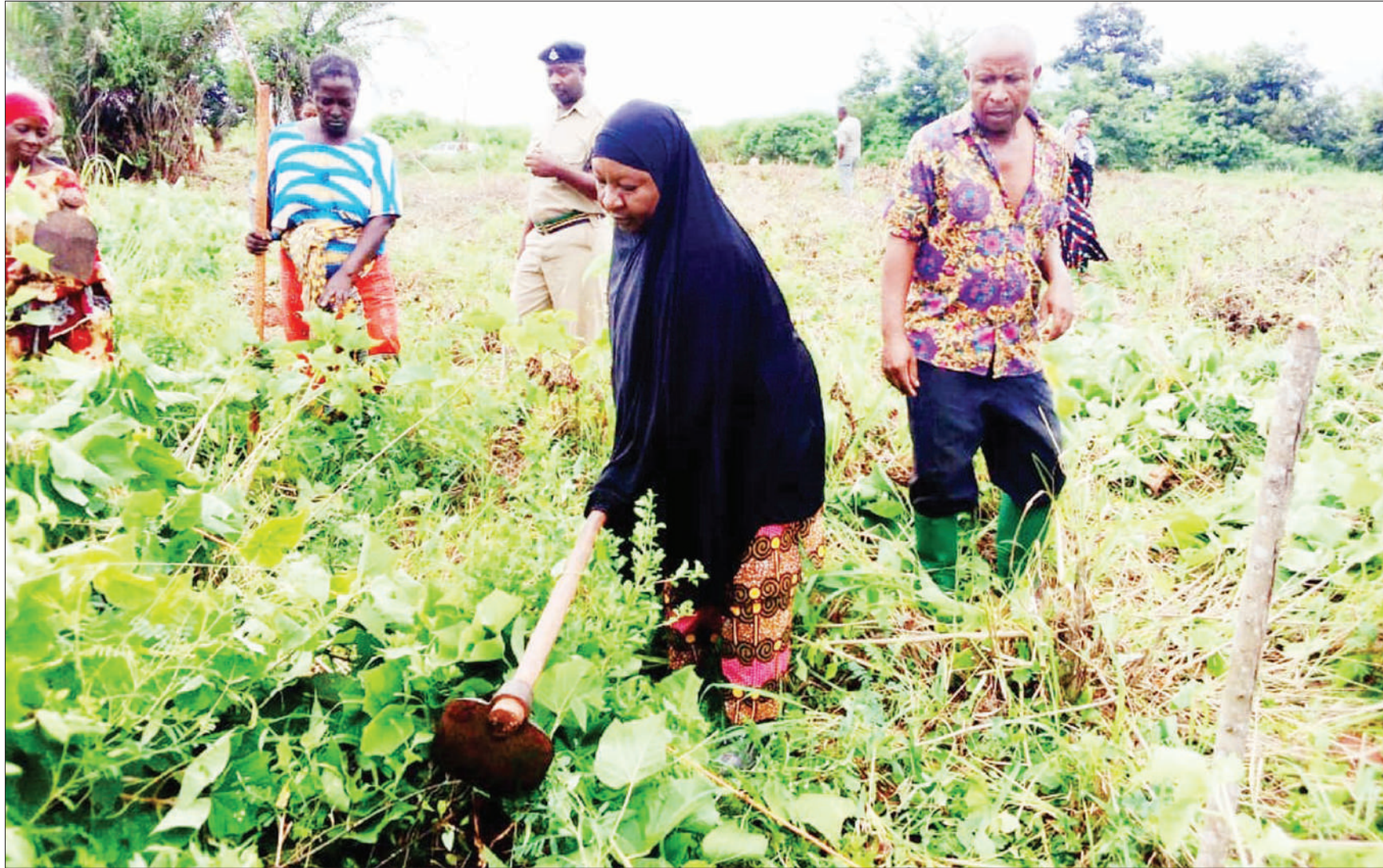
Muheza district commissioner Mwanasha Tumbo pictured yesterday helping in clearing the Upare site set aside for the construction of a village dispensary. Photo: Correspondent Steven William
