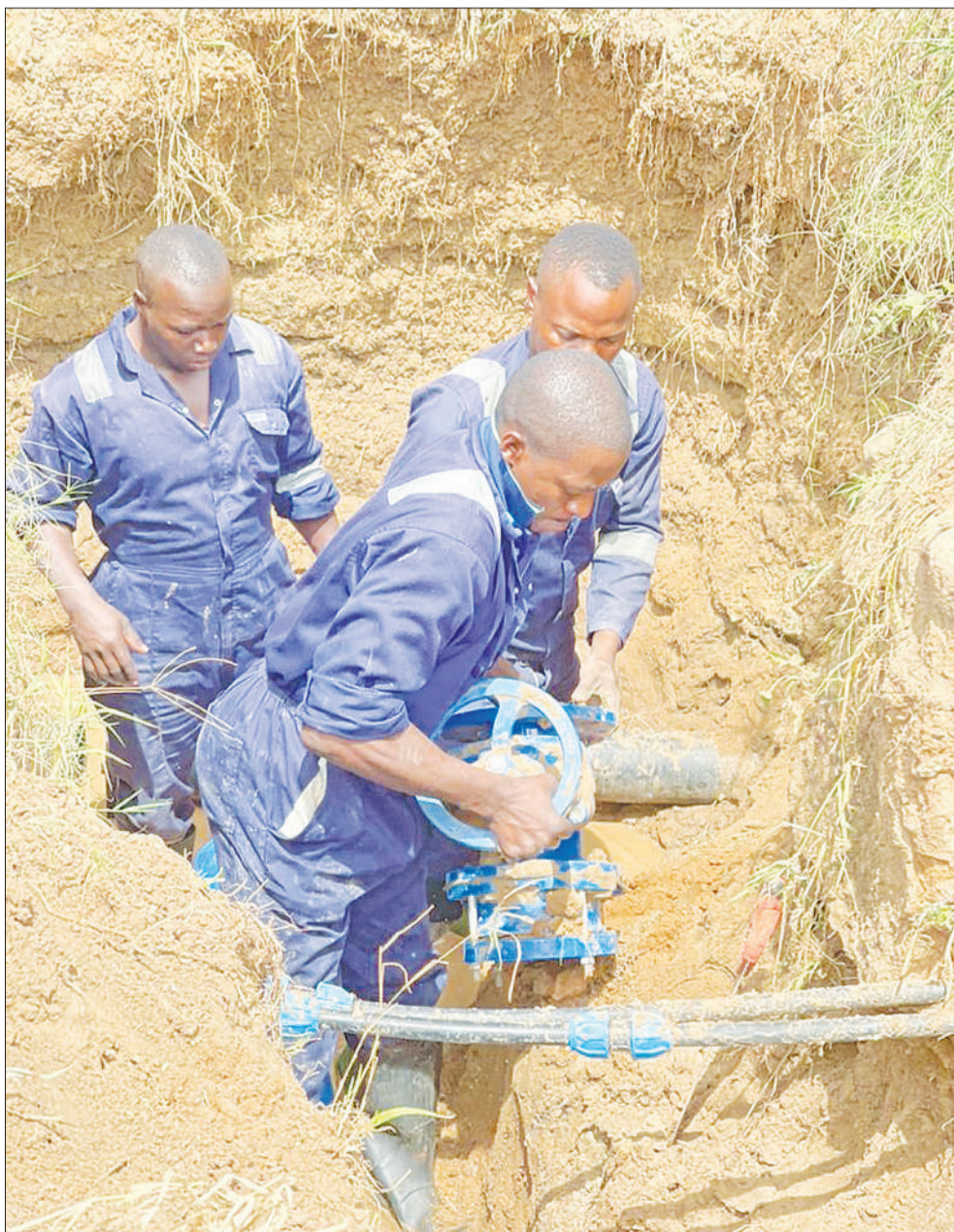
Technicians with the Dar es Salaam Water and Sanitation Authority (DAWASA) move to repair a leaking pipe in an effort to improve the supply of tap water at St Joseph Magengeni in Wazo ward, Dar es Salaam, yesterday. Photo: Correspondent Joseph Mwendapole
