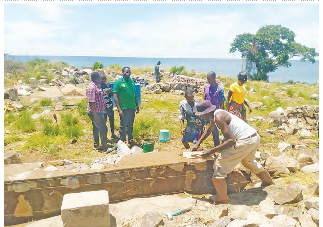
Residents of Rububa Island in Musoma Rural, Mara Region taking part in the construction of a foundation of one of the island's secondary classes recently. It is a strategy for the island to have its own secondary school to relieve their children of the inconvenience of crossing the river to pursue education. Photo: Correspondent
