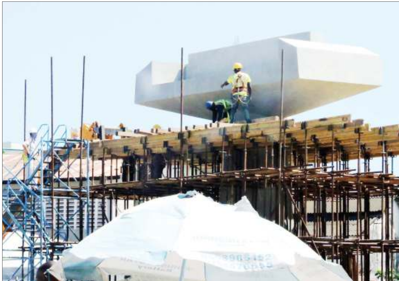
Tanzania Railway Corporation (TRC) employees at work during the construction of the Standard Gauge Railway - Ilala area in Dar es Salaam yesterday. Photo: Correspondent Getrude Mpezya
