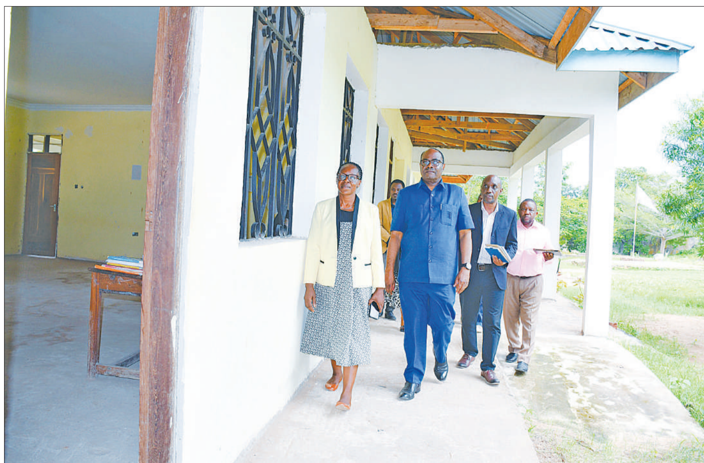
Tanzania Education Authority board chairman Dr Leonard Akwilapo (2nd-L) makes an inspection tour of progress in the construction of the Administration building at Lupaso Secondary School in Masasi District yesterday. Photo: Correspondent Joseph Mwendapole
