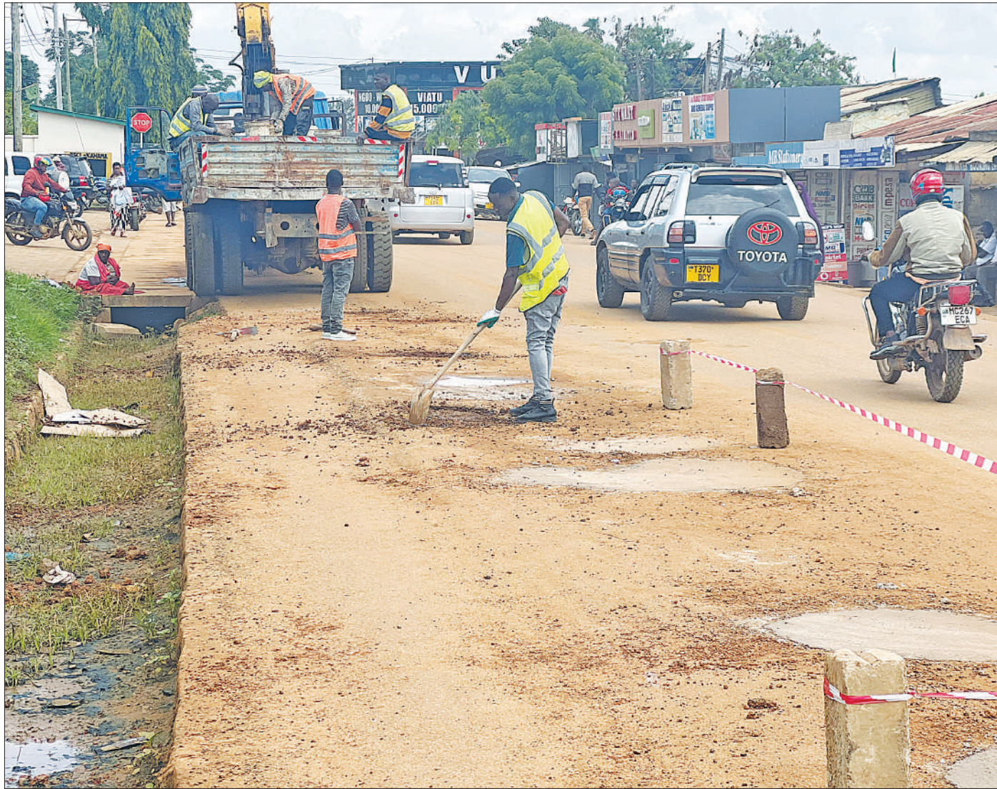
A potholed stretch of Lumelezi Road, which in part serves the Kahama town bus terminal, undergoes rehabilitation yesterday with World Bank funding. Photo: Correspondent Shaban Njia
