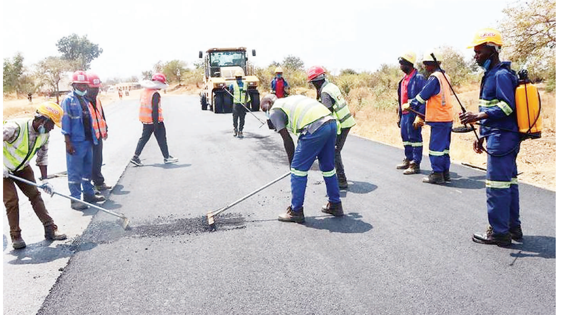
Photo taken on Aug. 27, 2024, shows asphalt pavement works on Malawi's M5 Road in Nkhotakota district, Malawi. Group/Handout via Xinhua)
