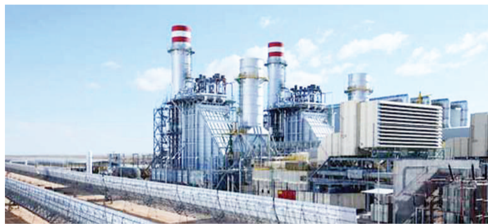
Ain Beni Mathar integrated combined cycle thermo-solar power plant, Morocco. Credit: Dana Smillie / World Bank. Photo ID: DS-MA111 World Bank
