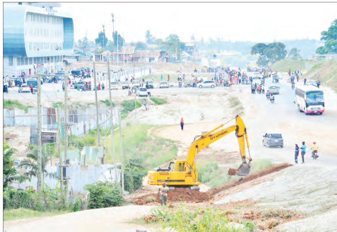
Caterpillar levels the ground for the road leading to Magufuli bus terminal situated at Mbezi - Mwisho in Dar es Salaam yesterday. Photo: Correspondent Miraji Msala
