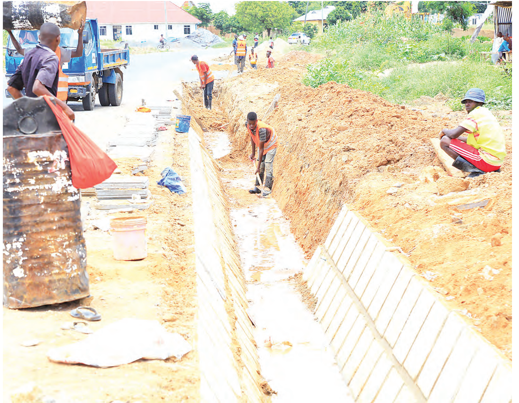
Construction of a trench gets under way beside Martin Luther Road at Swaswa in Dodoma, as captured yesterday. Photo: Correspondent Ibrahim Joseph
