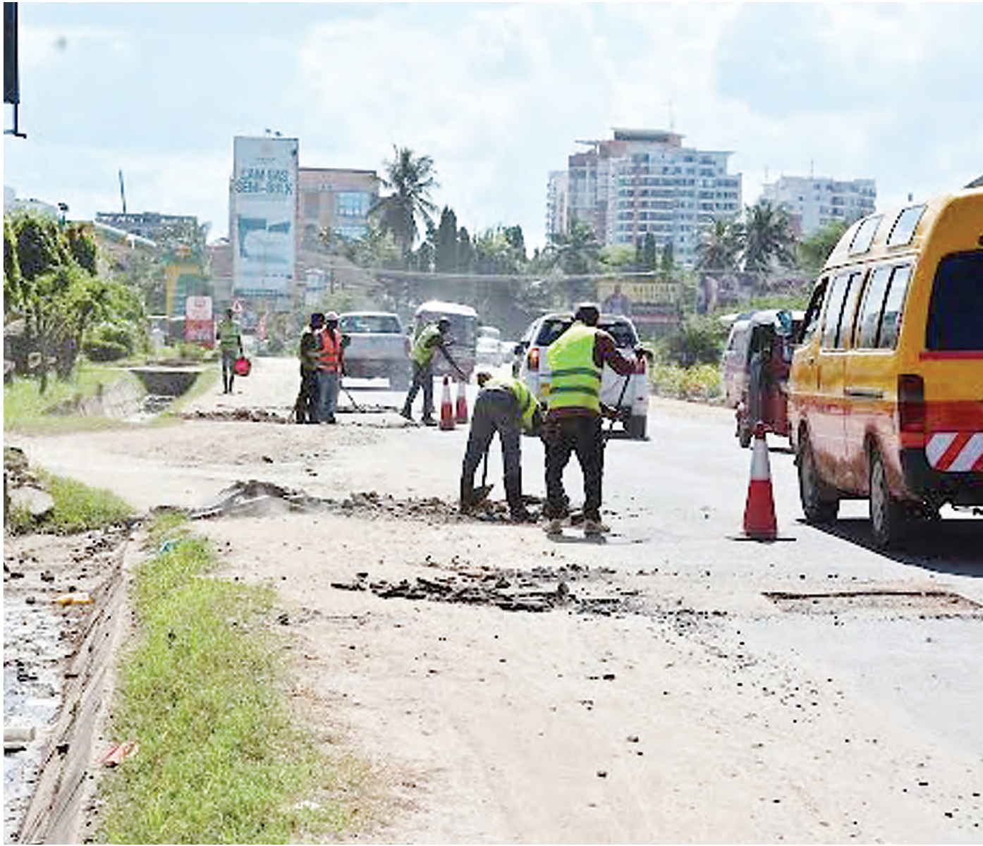
A Mikocheni section of Dar es Salaam's Mwai Kibaki Road undergoes rehabilitation yesterday. Photo: Correspondent Miraji Msala
