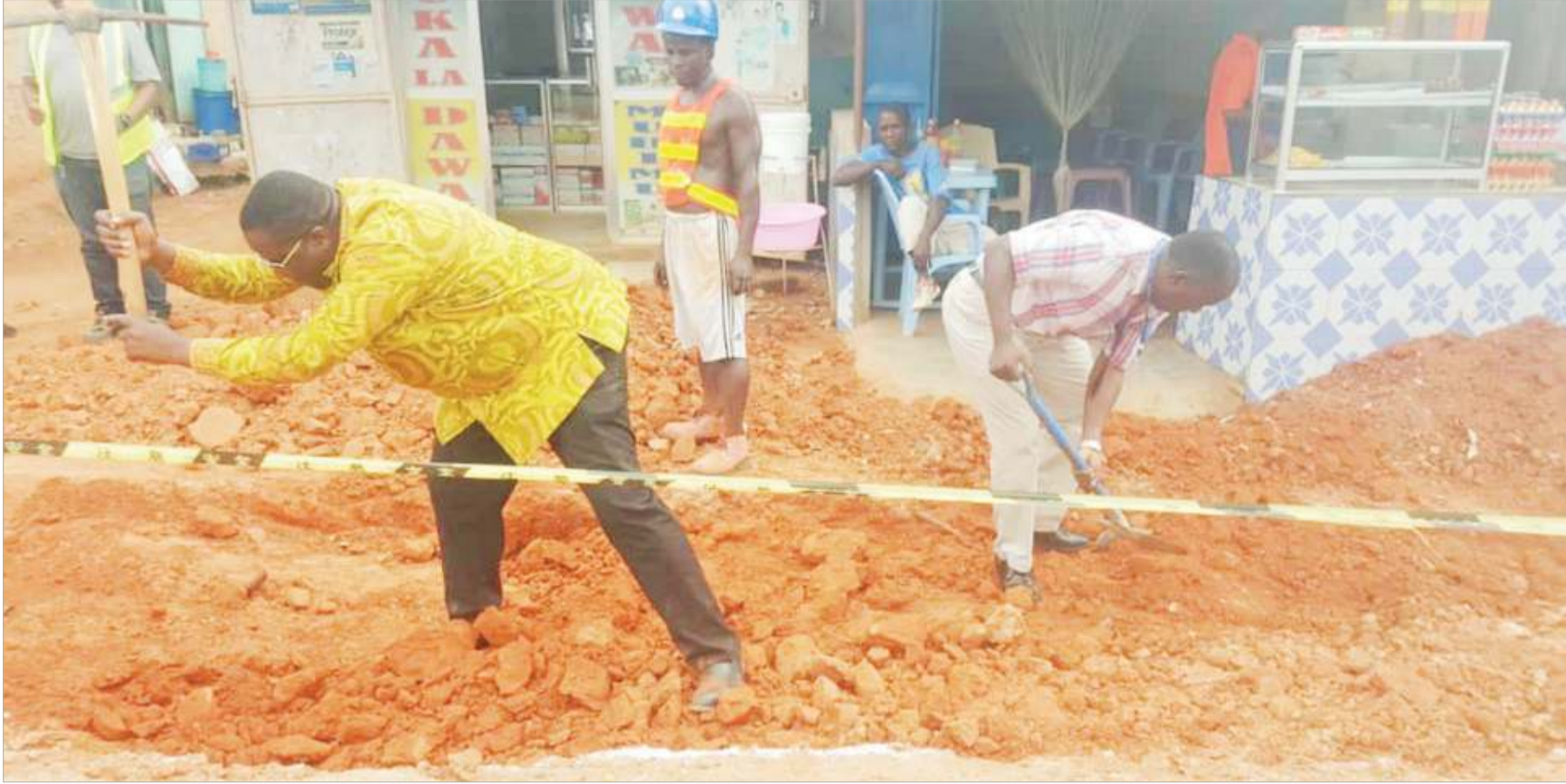
Dar es Salaam Water and Sewerage Authority (Dawasa) CEO Cyprian Luhemeja pictured yesterday participating in the digging of a waterway in Dar es Salaam's Mabwepande suburb, where the agency is laying water pipes. Photo: Guardian Correspondent
