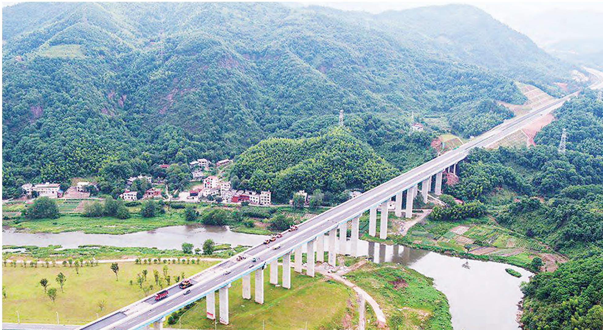
Construction workers pave asphalt on the surface of a super large bridge over the Pingshui River in Pingxiang, east China's Jiangxi province, August 11, 2021. The bridge is part of an expressway connecting the urban areas of Pingxiang city with Lianhua county of the city. File photo
