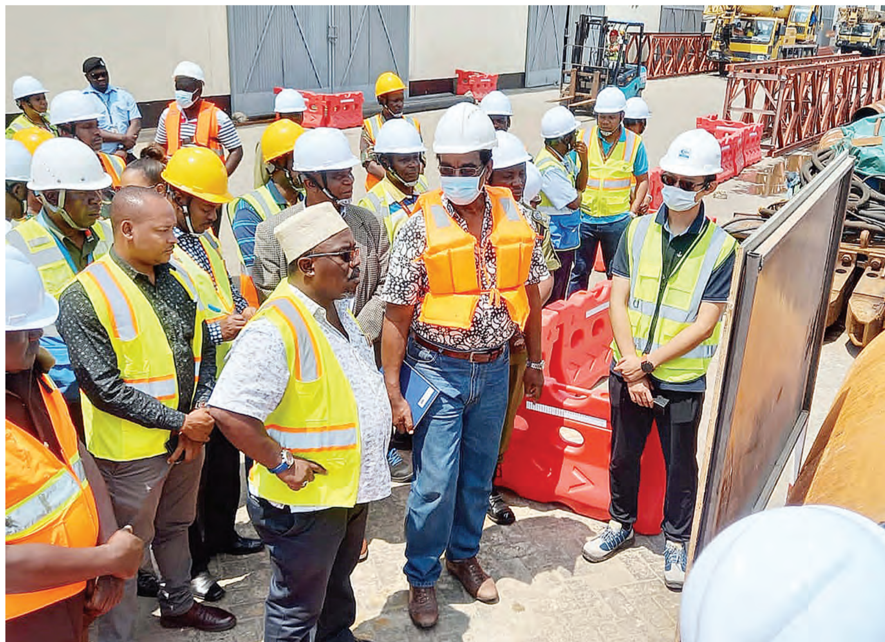
Tanga regional commissioner Adam Malima (foreground, in cap and glasses) makes an assessment tour of a pier undergoing construction at Tanga Port at the weekend. To his left is Tanga port manager Donald Ntaire. Photo: Correspondent Hamida Kamchala
