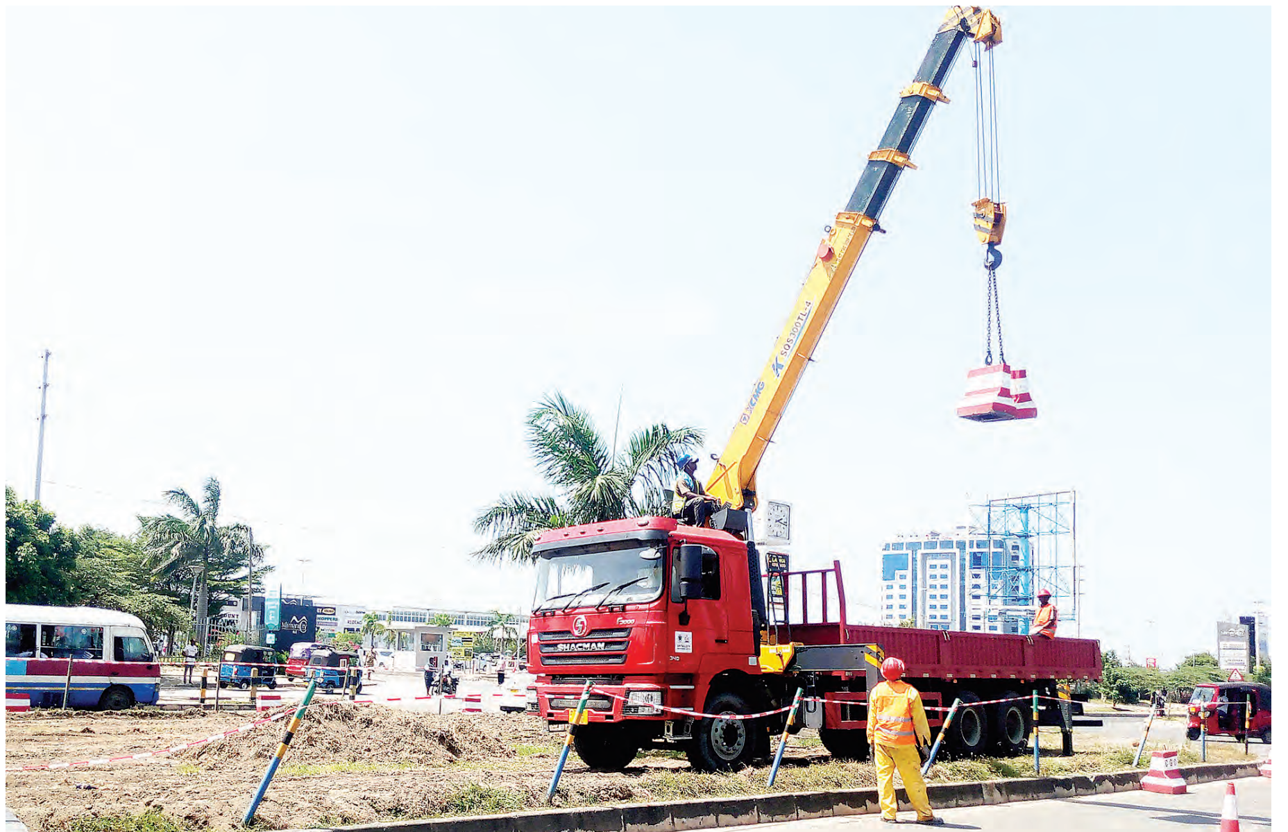
Preparations well under way yesterday for the implementation of the Bus Rapid Transit infrastructure project along the Mlimani City stretch of Dar es Salaam's Sam Nujoma Road. Photo: Correspondent Sabato Kasika
