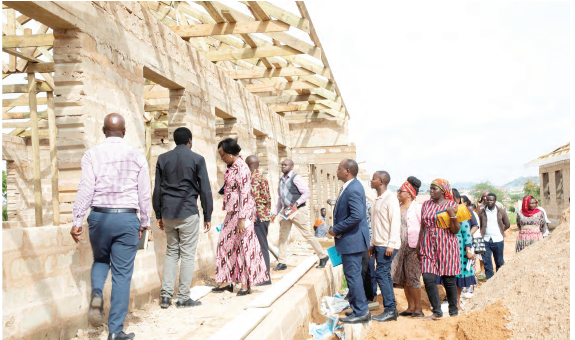
Dodoma regional commissioner Rosemary Senyamule (3rd-L) makes an assessment visit to a building under construction at Michese Secondary School in Mkonze ward, Dodoma Urban District, yesterday. Photo: Correspondent Peter Mkwavila
