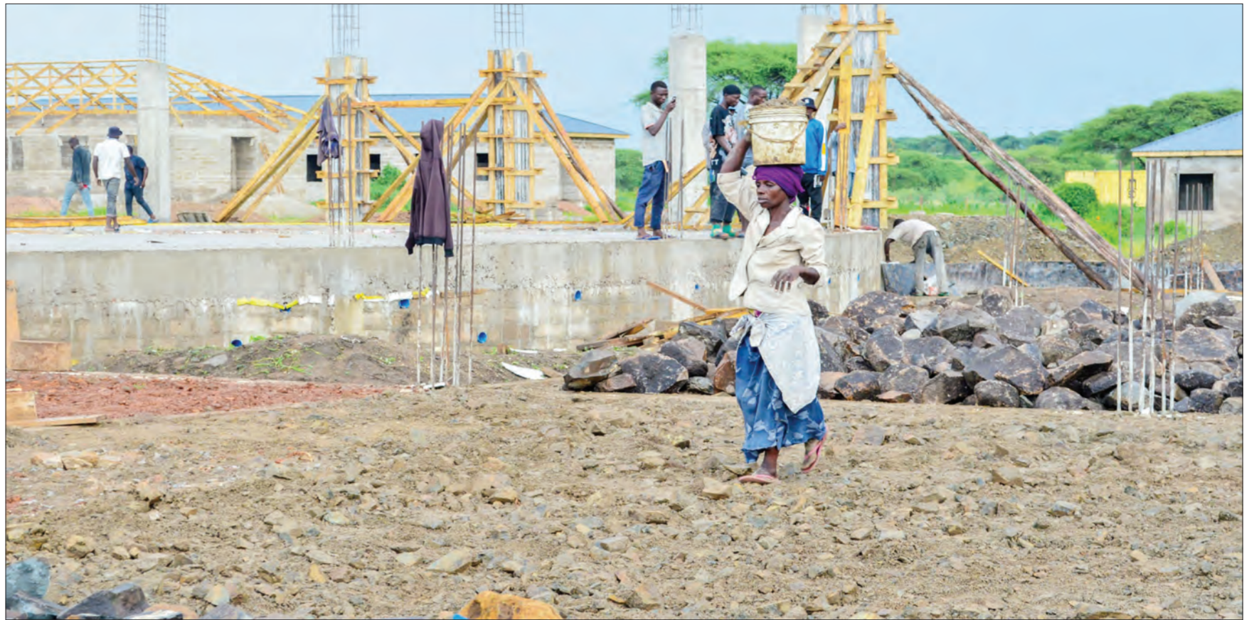
Residents of Bulamba village in Mara Region's Mwirara constituency take part in the construction of a building at a girls' secondary school on self-help basis, as found on Wednesday. Photo: Guardian Correspondent
