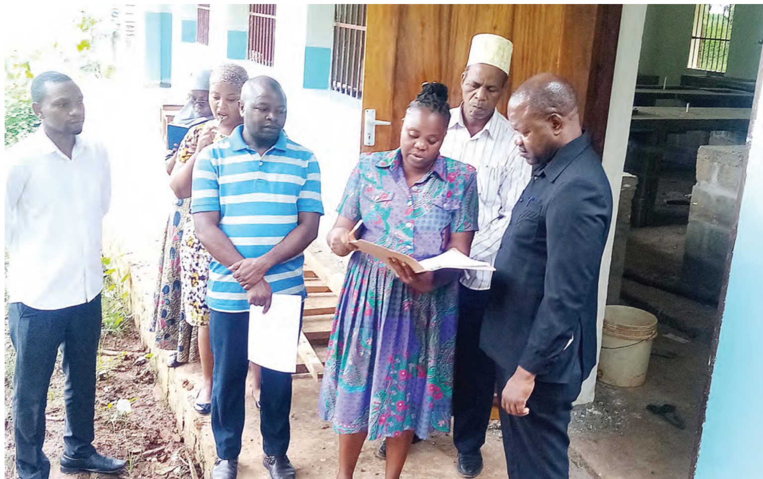
Neema Mapunda (2nd-R), headmistress of Mkurumuzi Secondary School in Muheza District, briefs Muheza district executive director Dr Jumaa Mhina (R) on Thursday on progress in the construction of a science laboratory building at the school. Photo: Correspondent Steven William
