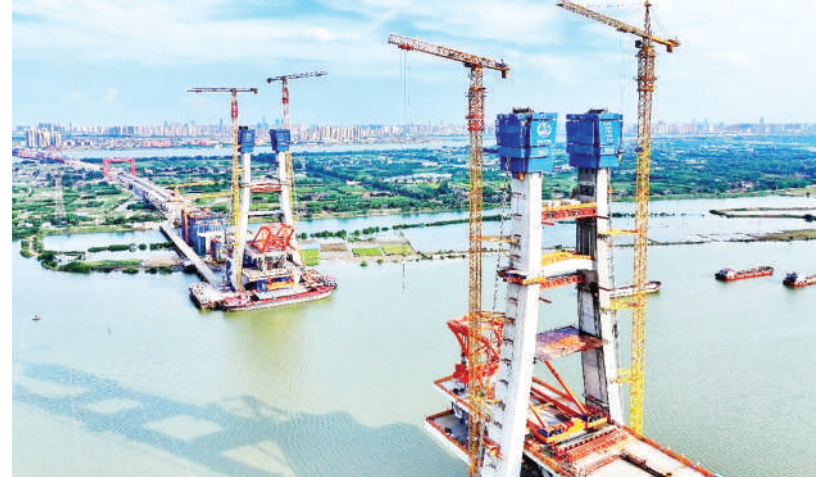
Photo shows the construction site of the Yangzizhou Ganjiang Highway-Railway Bridge in east China's Jiangxi province. (Photo by Zhu Haipeng/ People's Daily Online)
