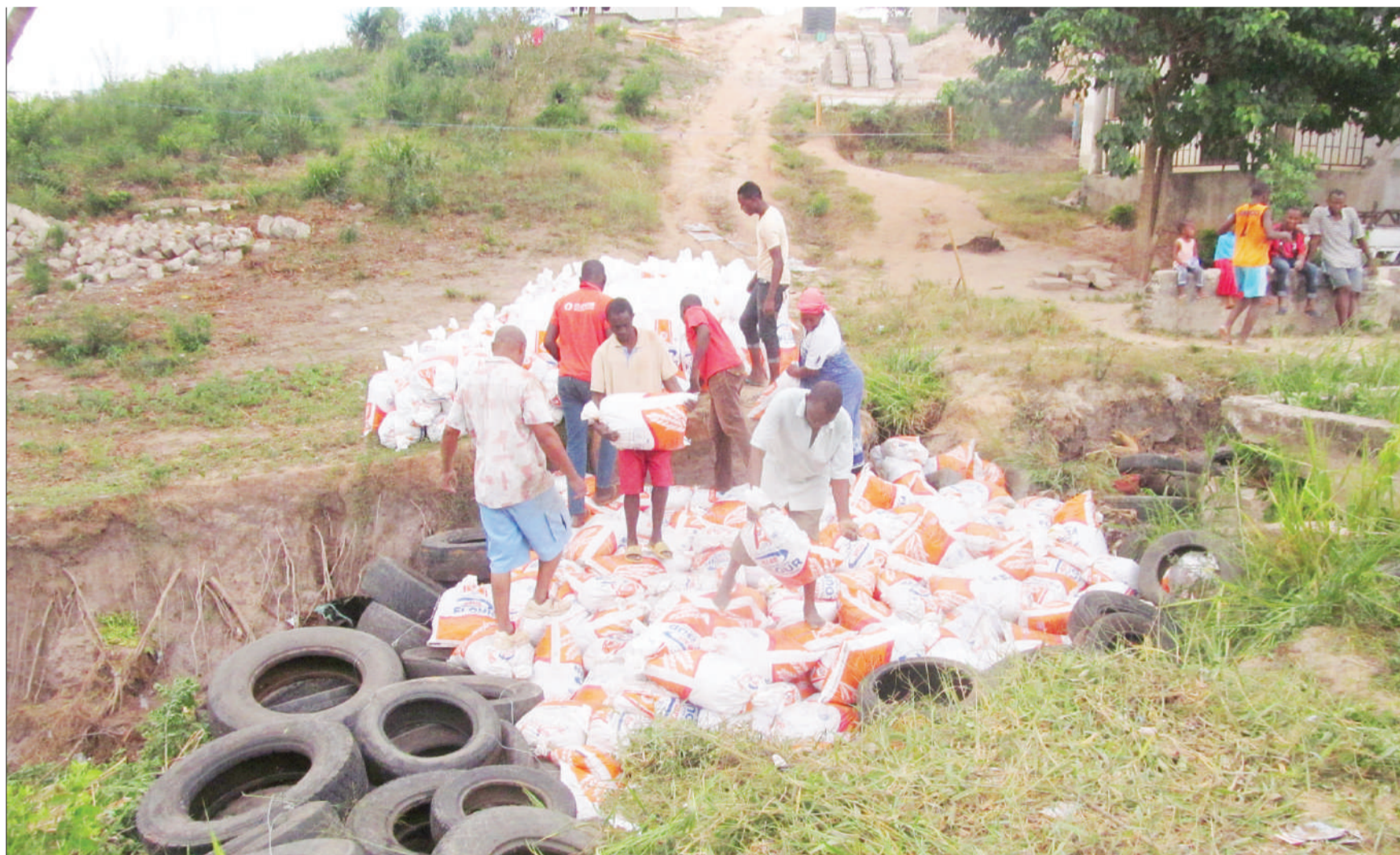
Residents of King'azi B at Kwembe in Kinondoni District, Dar es Salaam, in a desperate move to repair a dust-road badly damaged by recent rains, as found yesterday. Photo: Correspondent Sabato Kasika
