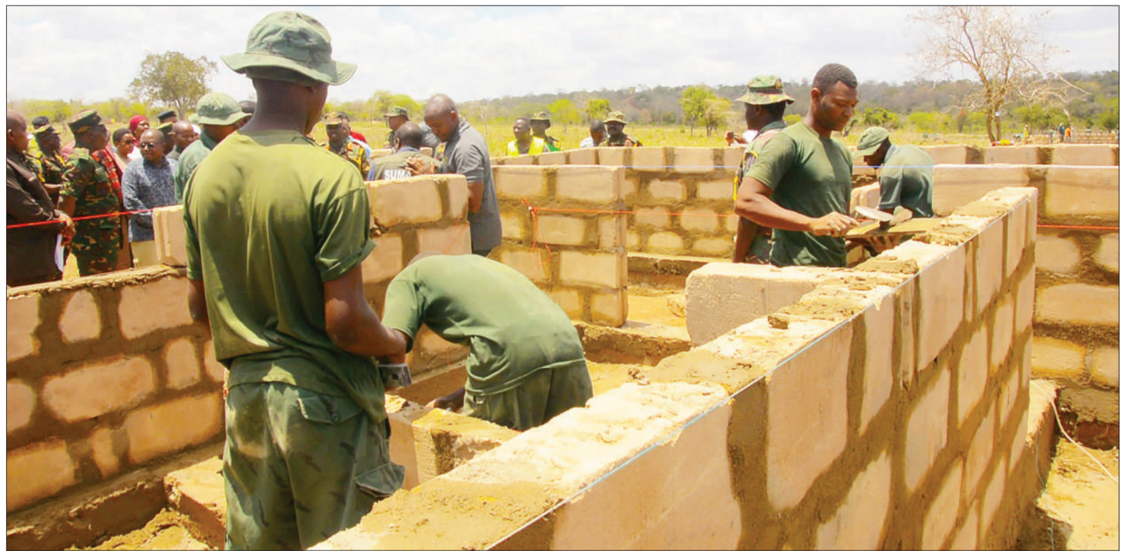
Members of the National Service corps construct houses for Ngorongoro National Park residents who have shifted voluntarily to Msomera in Handeni District, Tanga Region yesterday. Photo: Correspondent Hassan Mabuye
