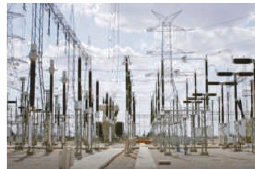
Iringa - Shinyanga Backbone Transmission Project
