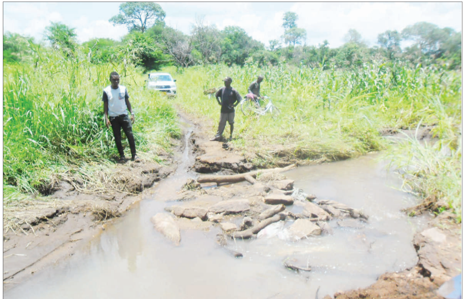
This is Nalingwenya river, which traverses Mkong'ondela village in Mtwara Region's Nanyumbu District and across which the Tanzania Rural and Urban Roads Agency (Tarura) is planning to build a bridge to link Michiga and Makong'ondela villages. The scene was captured yesterday. Photo: Guardian Correspondent
