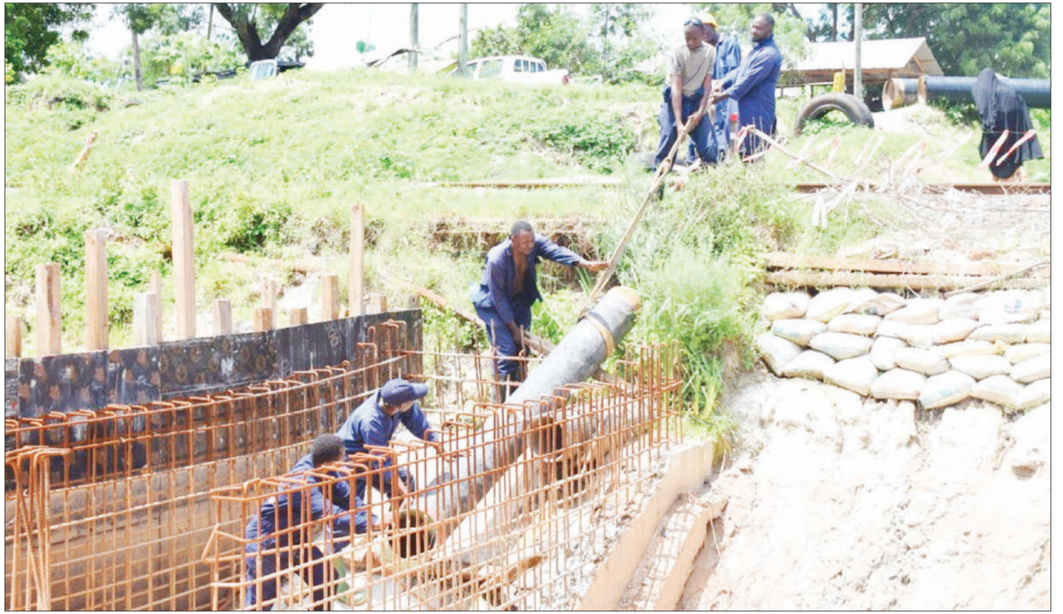
Dar es Salaam Water and Sanitation Authority technicians pictured in the city's Vingunguti suburb yesterday moving to rehabilitate a main water pipe swept away by recent rains. The pipe serves Kimanga, Kisukuru Chini, Chama, Liwiti, Chang'ombe, Barakuda Ugombolwa, Segerea, Mwembeni, Mpera and Zimbili 'A' suburbs. Photo: Guardian Correspondent
