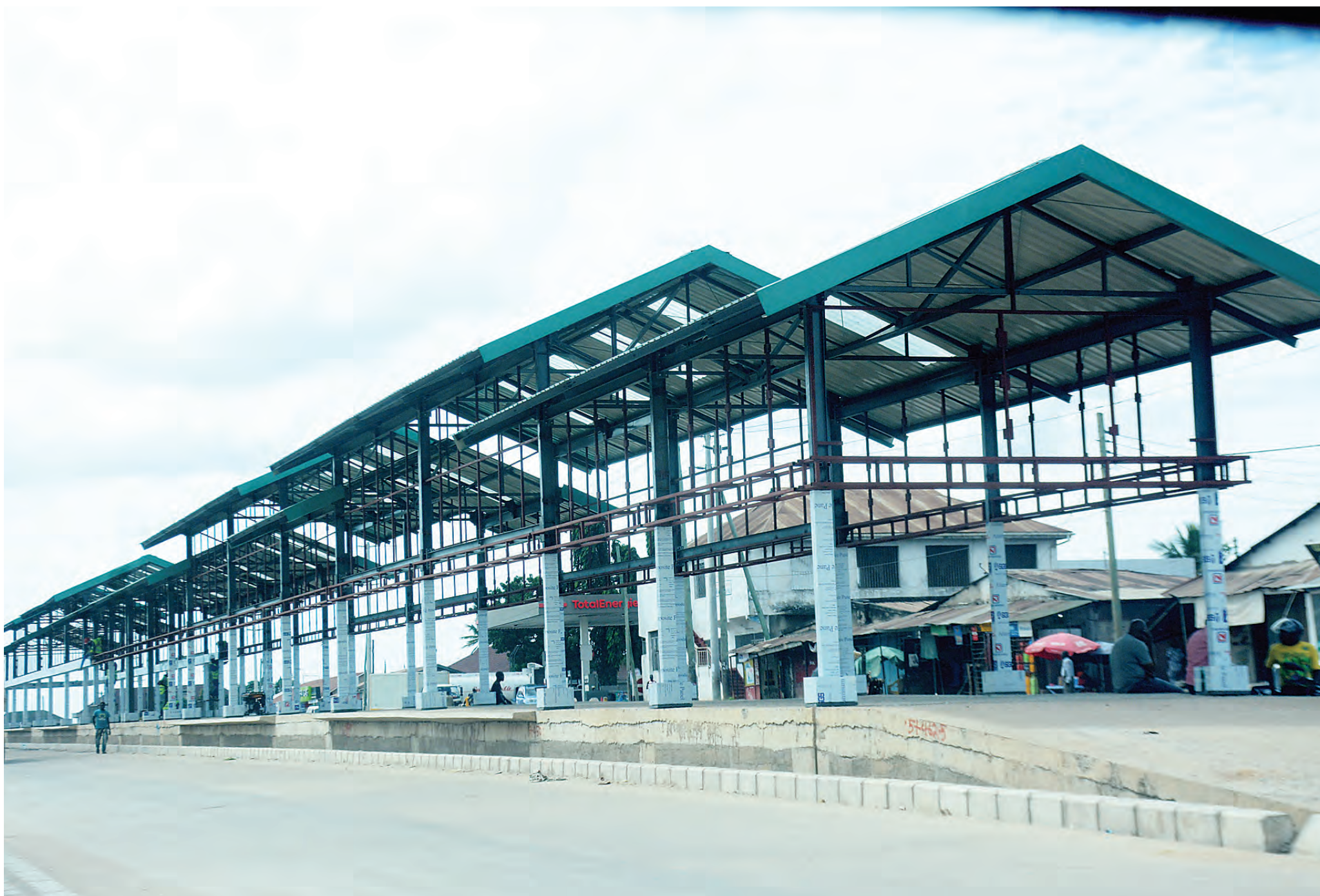
A view captured yesterday of the Mtoni Mtongani Bus stop, as captured yesterday. The stop is undergoing construction at a section of Kilwa Road under Phase Two of the Dar es Salaam bus rapid transit (DART) project. Photo: Correspondent Jumanne Juma
