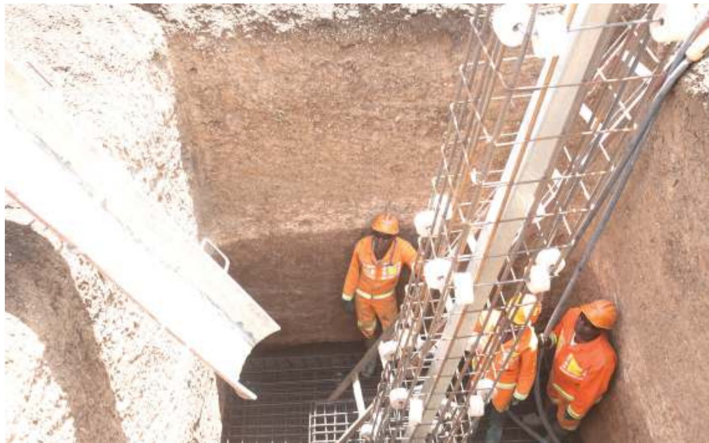
Some of technicians from Bouygues Energy and Service readies to put concrete when building a foundation for a 400kV electric tower near Nanja village in Arusha recently. The company is part of three companies entrusted by TANESCO to construct a 500km power transmission line from Singida to Isinya in Kenya. The project assured large and small manufacturers of reliable power supply. PHOTO - FINANCIAL TIMES CORRESPONDENT.
