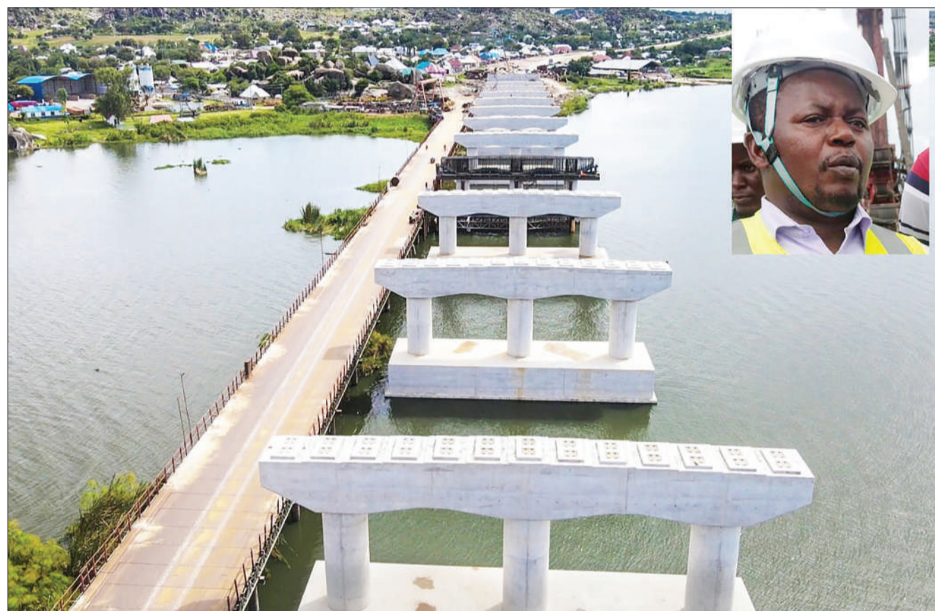
This is a view of Kigongo-Busisi Bridge in Mwanza Region, as captured at the weekend. According to Tanzania National Roads Agency (Tanroads) CEO Rogatus Mativila (inset), construction has reached 72 per cent. Photo: Guardian Correspondent
