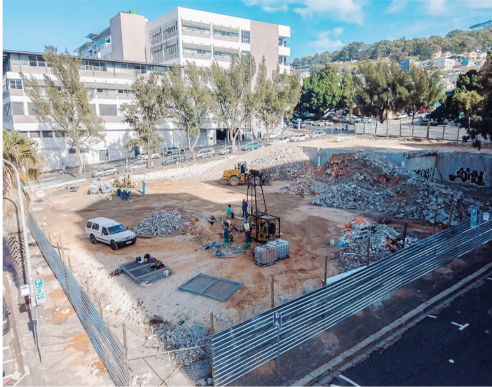
Demolition of the old structure is near completion and recyclable materials have been saved for reuse
