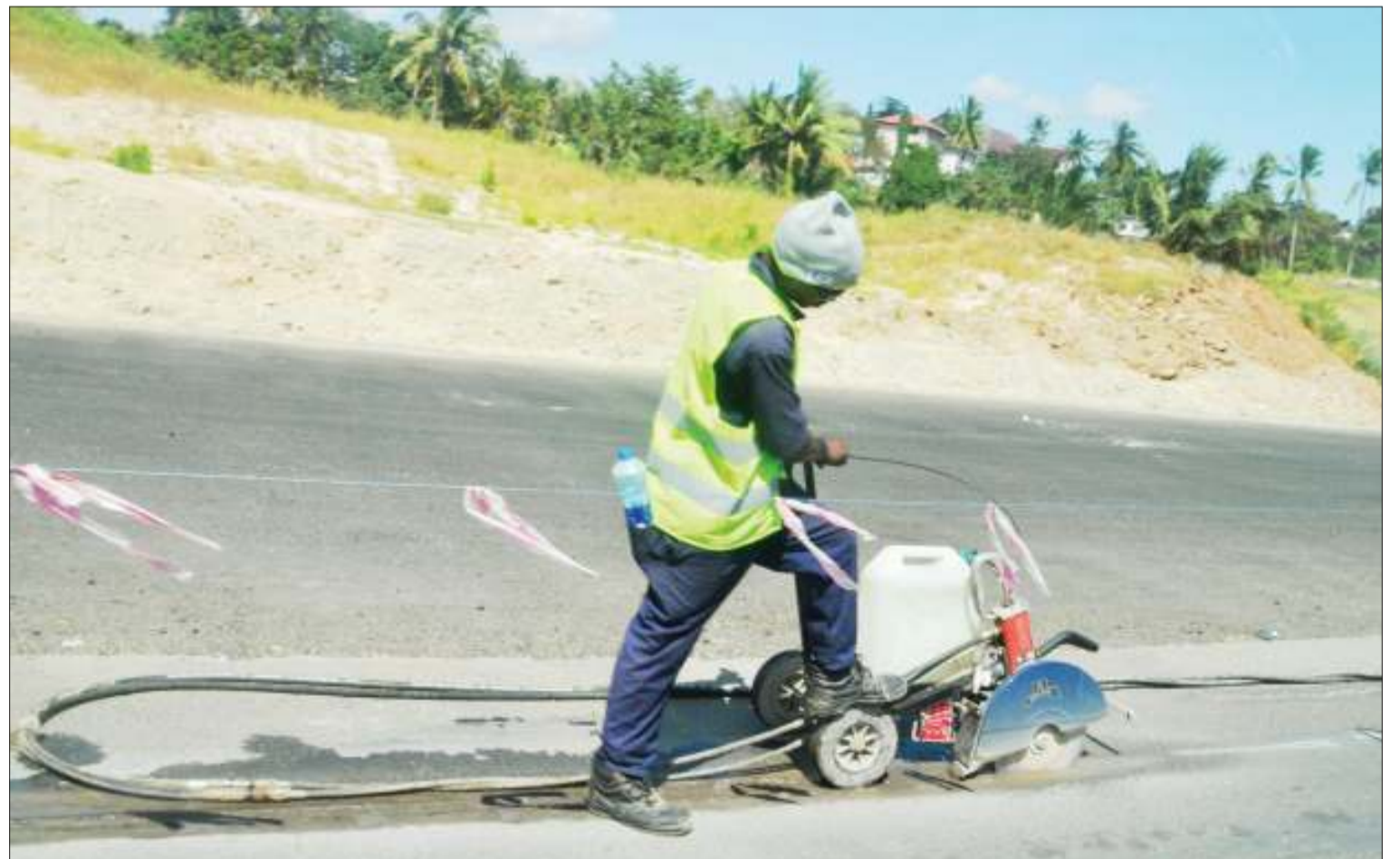
An Estim construction firm worker plays his part in the ongoing first-phase expansion of the stretch of Morogoro Road running from Dar es Salaam suburb Kimara to Kibaha in Coast Region into a six-lane dual carriageway, as captured at Kimara Stop Over yesterday. Photo: John Badi
