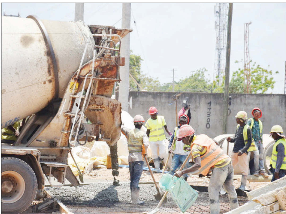
Construction of the Bus Rapid Transit infrastructure in progress along the Kurasini stretch of Dar es Salaam's Kilwa Road yesterday. Photo: Correspondent Jumanne Juma
