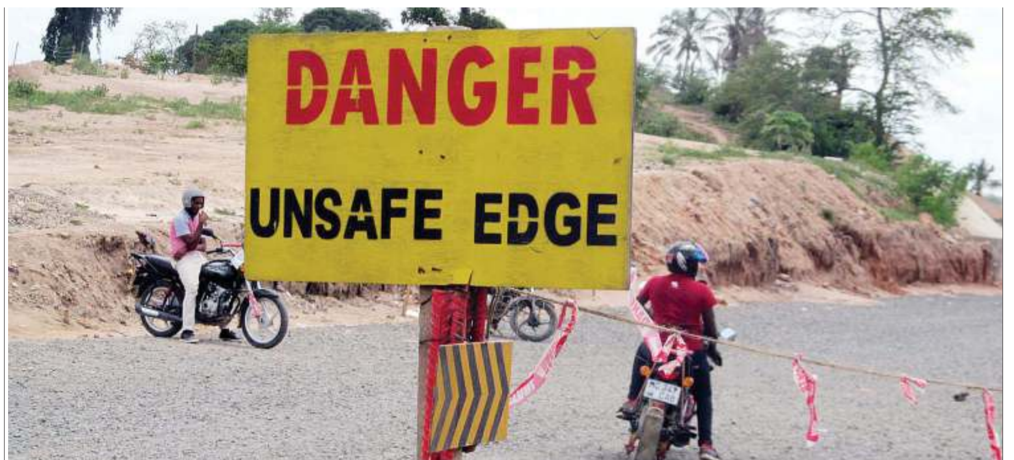
A self-explanatory but largely ignored sign post installed at Kimara Stop-over in Dar es Salaam to caution motorists with respect to the ongoing expansion of Morogoro Road, as captured yesterday. Photo: Correspondent Sabato Kasika
