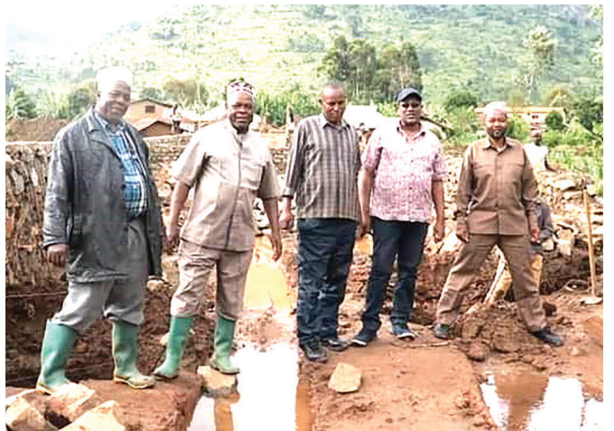
Lushoto district commissioner Kalist Lazaro (2nd-R) accompanied by Dule and Mwangoi ward officials when inspecting progress in the construction of Majulai-Mesa road, with the ongoing rains proving a clear obstruction. Photo: Correspondent Steven William
