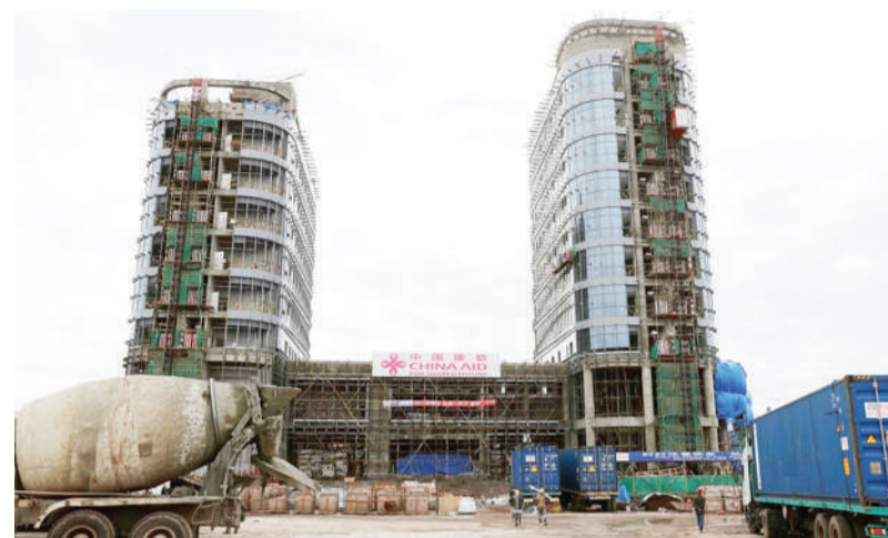
Photo taken on Aug. 16, 2022, shows the construction site of the Headquarters Building Phase I Project of the Africa Centers for Disease Control and Prevention (Africa CDC) in Addis Ababa, Ethiopia. File photo
