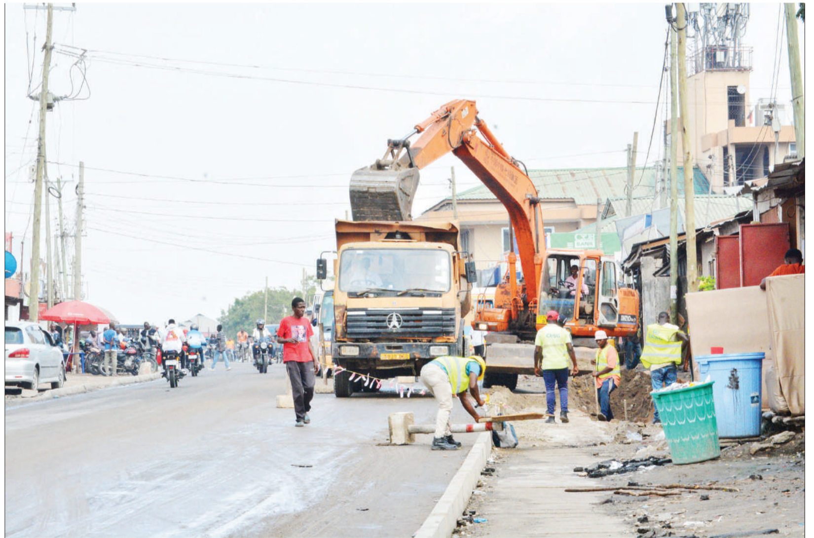
Technicians at work constructing rain water harvesting trench along Kinondoni-Mwanayamala road in Dar es Salaam yesterday.
