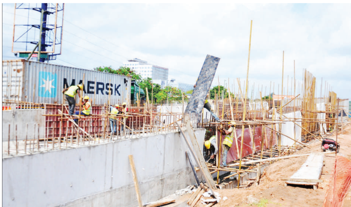
Technicians at work. More road projects soon to ease Dar's traffic congestion. Chang'ombe and Nyerere flyover in progress. Photo: Correspondent Jumanne Juma
