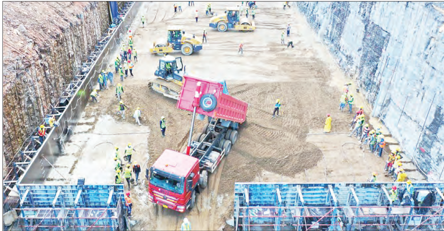
Construction work going on at Julius Nyerere Hydro Power Project along River Rufiji.
